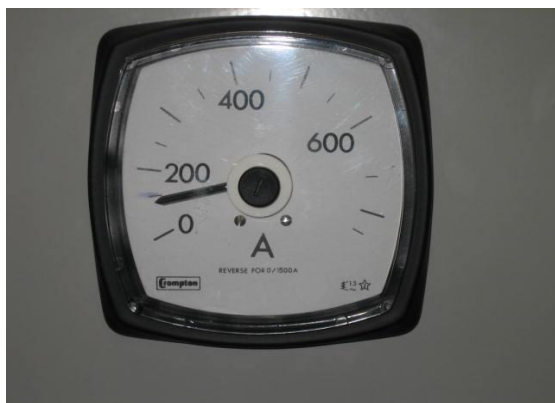
Figure 5 A switchgear ammeter
