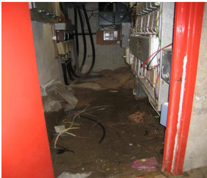
Figure 1 - Water Ingress to the Metering Installation rendering it unsafe to access the Metering Equipment
