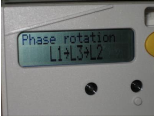
Figure 1 – Non-Standard Phase Rotation via Settlement Meter display.
